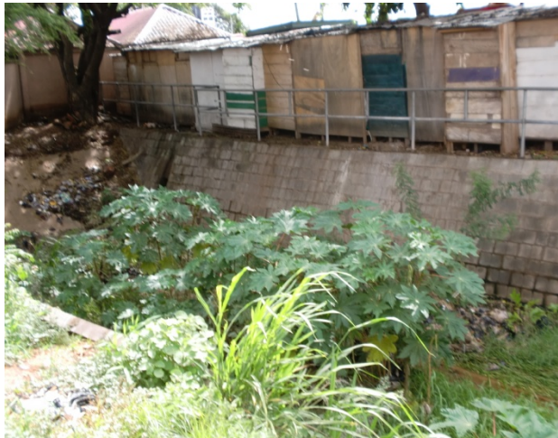
Fig 6.5: Gutter choked with weeds & grasses in Odawna Pedestrian market, Accra
