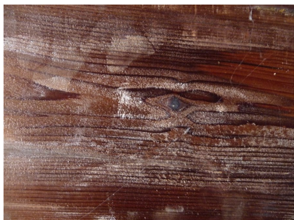
Fig. 2 Efflorescence on the ceiling of Aspaas House in the second floor
