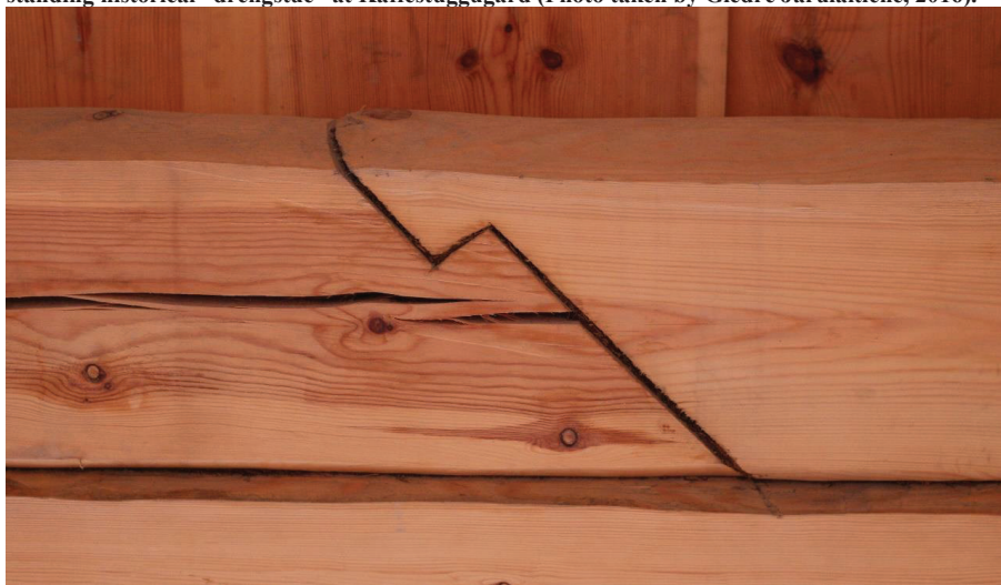
Figure 122. A newly-reproduced hooked scarf joint (skrå hakeskjøt) in the outbuilding (Photo taken by Giedrė Jarulaitienė, 2016).
