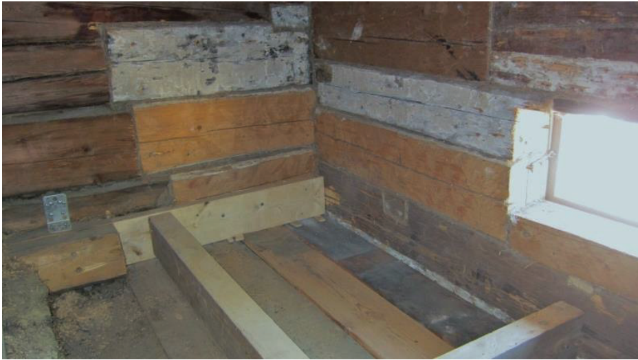
Figure 188. The rotten corner was fixed with re-used logs from various demolished buildings. (Photo taken by Giedrė Jarulaitienė, 2011).
