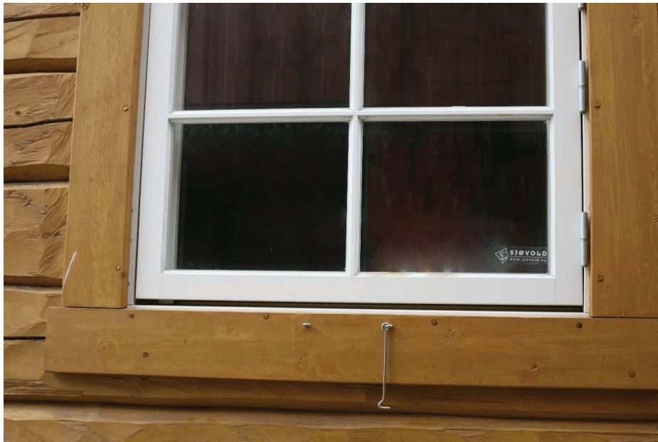
Figure 138. A window of the new outbuilding – as advertisement of the local factory, producing windows and doors in traditional appearance (see the chapter above “Initiatives of the field of heritage conservation, which ended up serving the field of building industry”). (Photo taken by Giedrė Jarulaitienė, 2016).
