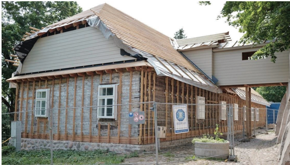
Figure 206. The restoration of the 19 th century Rectory next to the Catholic Parish Church and the reconstruction of the closed corridor over the street (Photo taken by Giedrė Jarulaitienė, 2019).
