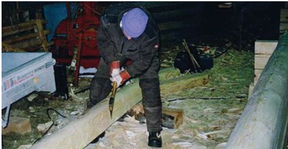
Figure 119. The hewing of external side of logs for the new outbuilding (The photographer unknown, 2009. The private archive of the carpenter).
