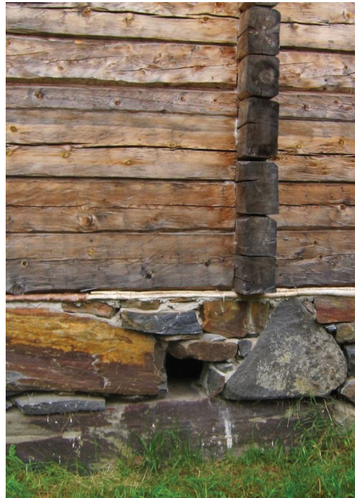
Figure 181. The precise application of traditional workmanship at Linnusperä in Kokkola. (Photo taken by Giedrė Jarulaitienė, 2011).
