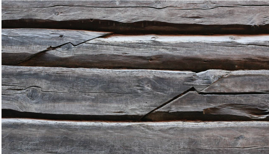
Figure 121. Old hooked scarf joints (skrå hakeskjøter), visible on the external façade of the nearby standing historical “drengstue” at Kaffestuggugård (Photo taken by Giedrė Jarulaitienė, 2016).
