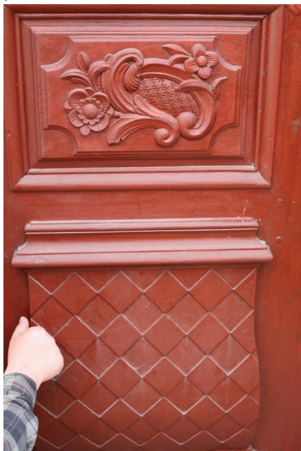
Figure 67. A carpenter's observation of the attached wooden carving on the front façade of the main door at P. P. Hiort's funeral chapel. (Photos taken by Giedrė Jarulaitienė, 2016)
