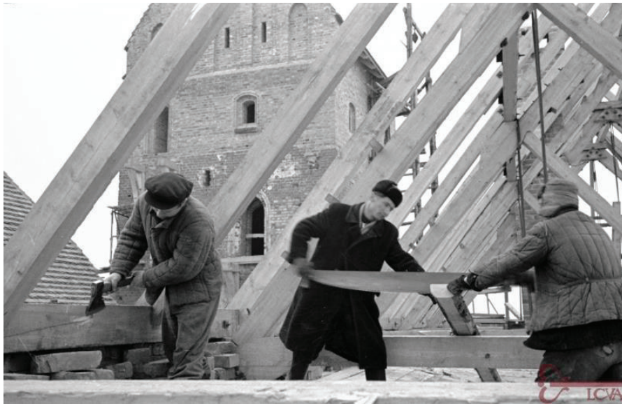
Figure 227. The process of restoration and reconstruction of Trakai Island Castle. The restoration team was composed of (left to right) the “brigadier” Z. Morkevičius and the carpenters Petras Karpavičius and Vladas Karpavičius. (Photo taken by V. Bražas and M. Baranauskas, 1960. Central State Archives of Lithuania, 0-013246).
