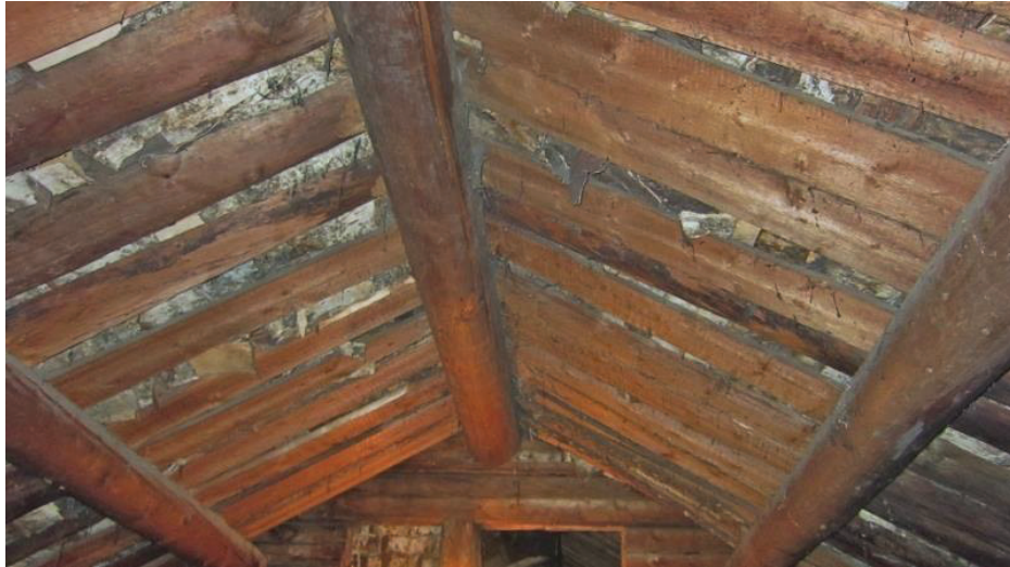
Figure 187. The original structural part of the roof and the authentic insulating layers of birch bark were left intact under the newly-covered roof with tin-plates. (Photo taken by Giedrė Jarulaitienė, 2011).
