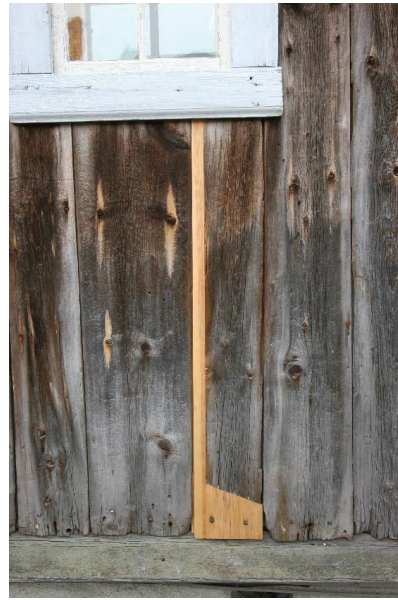
Figure 71. The gradual recent changes of the damaged parts of panelling at Per Amundsagården (Photo taken by Giedrė Jarulaitienė, 2011).
