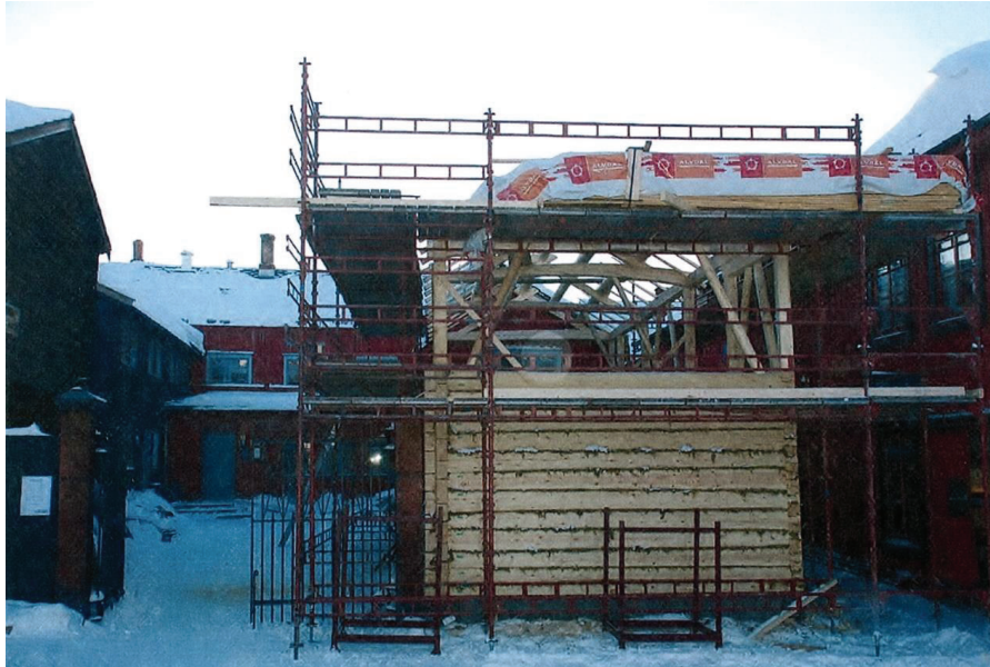
Figure 129. The process of assembling the ready-made logs at the site (Photographer unknown, 2008, The private archive of the carpenter).
