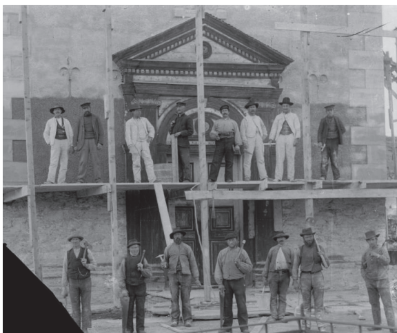
Figure 46. Imitations of ashlar masonry in the corners of the church tower at Røros were concealed under the renovation works in 1904. The original lime mortar was replaced with cement-containing plaster (Brønne, 2003, 15). (Photo taken by Iver Olsen, 1904, ©Røros museet, RMUB.251781).
