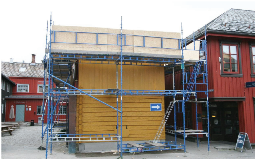
Figure 130. The final phase of the construction – the roof covering (Photo taken by Giedrė Jarulaitienė, 2009).
