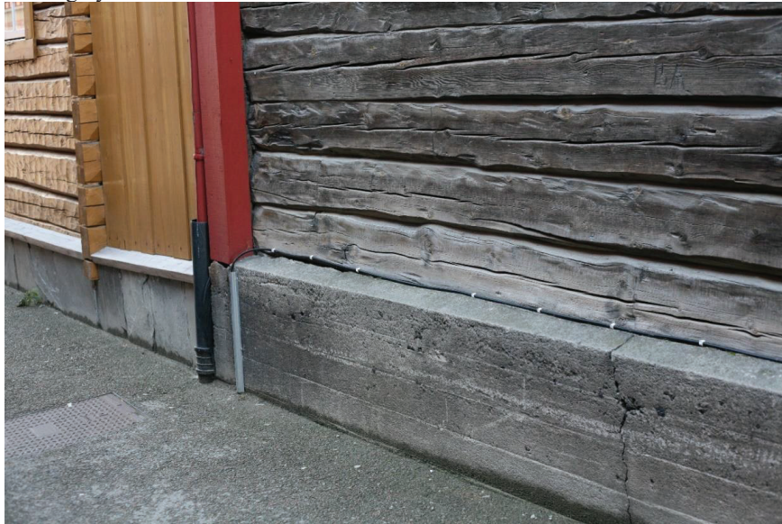
Figure 59. The modern solution - the concrete patched on foundations of the historical wooden building at Kaffestuggugård . (Photo taken by Giedrė Jarulaitienė, 2016)
