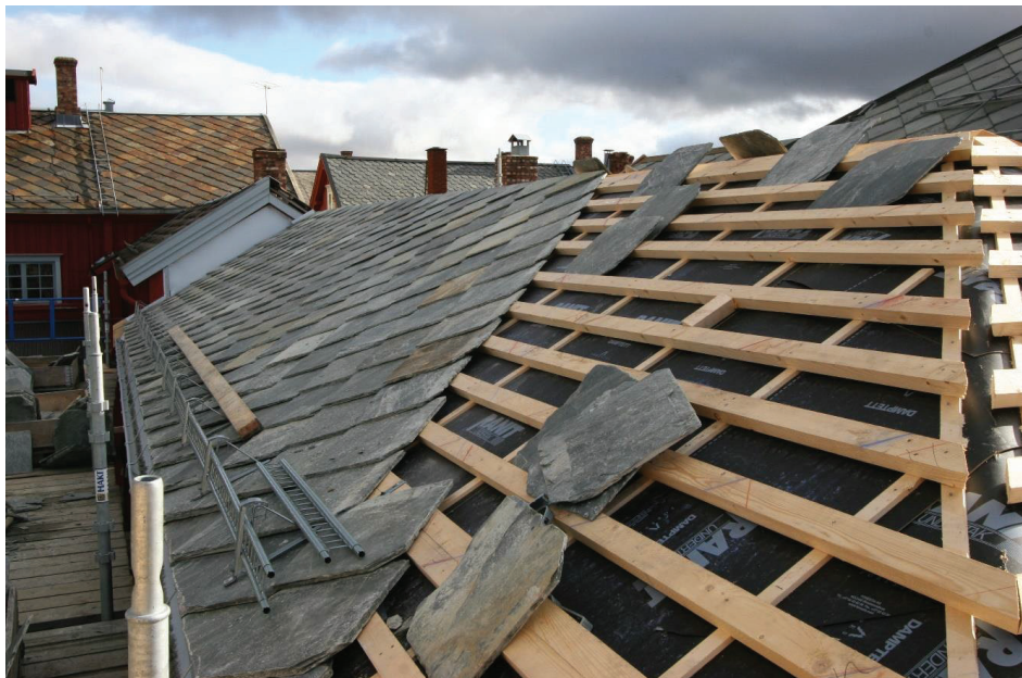
Figure 137. The roof covering of the outbuilding at Kaffestuggugård with local slates (Photo by Giedrė Jarulaitienė, 2009).
