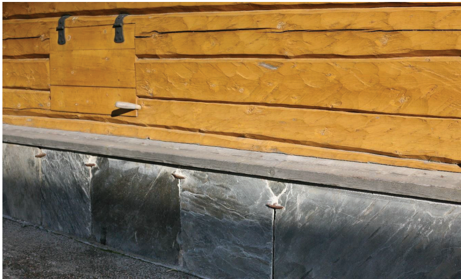
Figure 133. The hidden concrete foundation under traditional stone slates, fastened with forged spikes (Photo by Giedrė Jarulaitienė, 2016).
