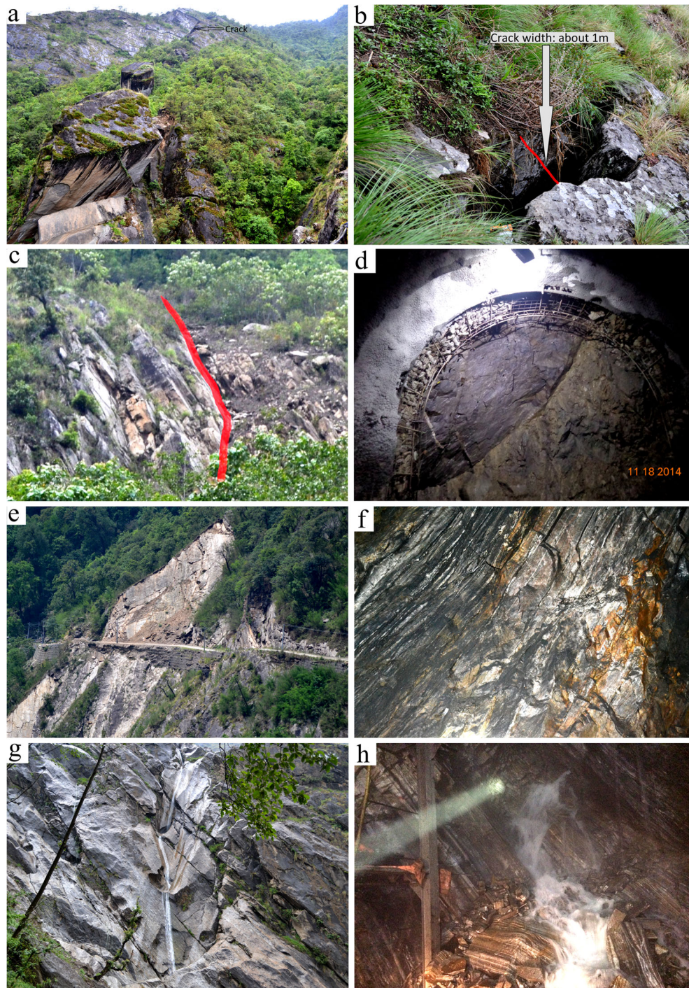
Fig. 15 a Big boulders and open cracks seen on the surface (photo 4 in Fig. 10a); b Approx. 1 m wide crack seen on the surface (photo 6 in Fig. 10b); c Typical weakness zone at surface (photo 5 in Fig. 10b); d Weakness zone at the HRT (photo credit: UTHP); e Typical weathering condition of rock mass at surface; f Typical weathering condition inside tunnel; g Typical rivulet at surface topography at about tunnel level (photo 2 in Fig. 10a); h concentrated tunnel inflow of about 1500 l/min at 7 + 487 m chainage inside the HRT (Photo credit: UTHP)
