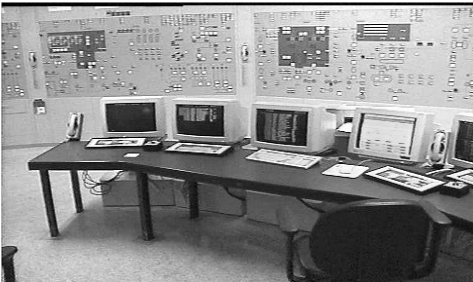
Figure 2. Turbine side of the Swedish Forsmark 3, illustrating a hybrid solution where the monitors in front are used for information gathering and the panels in the back are used for both monitoring and operation.
