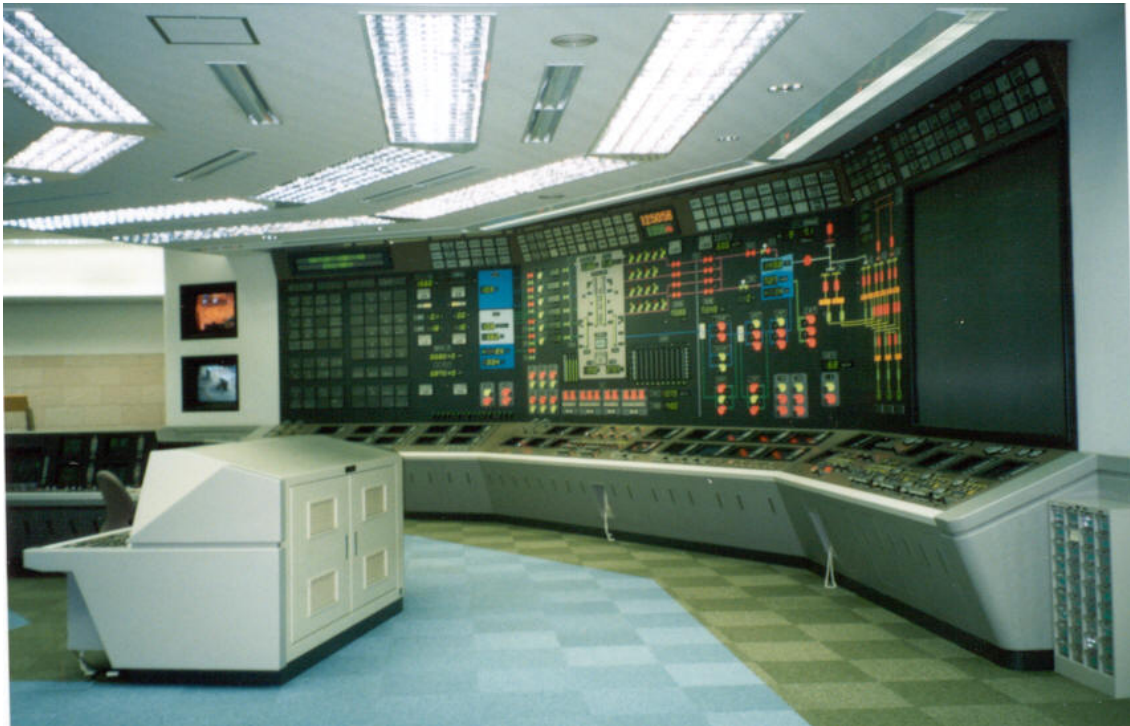
Figure 3. Kashiwazaki unit 6, Japanese advanced NPP control room. Most control panels are replaced with large screen information panels and the process is controlled from the operators workstations.
