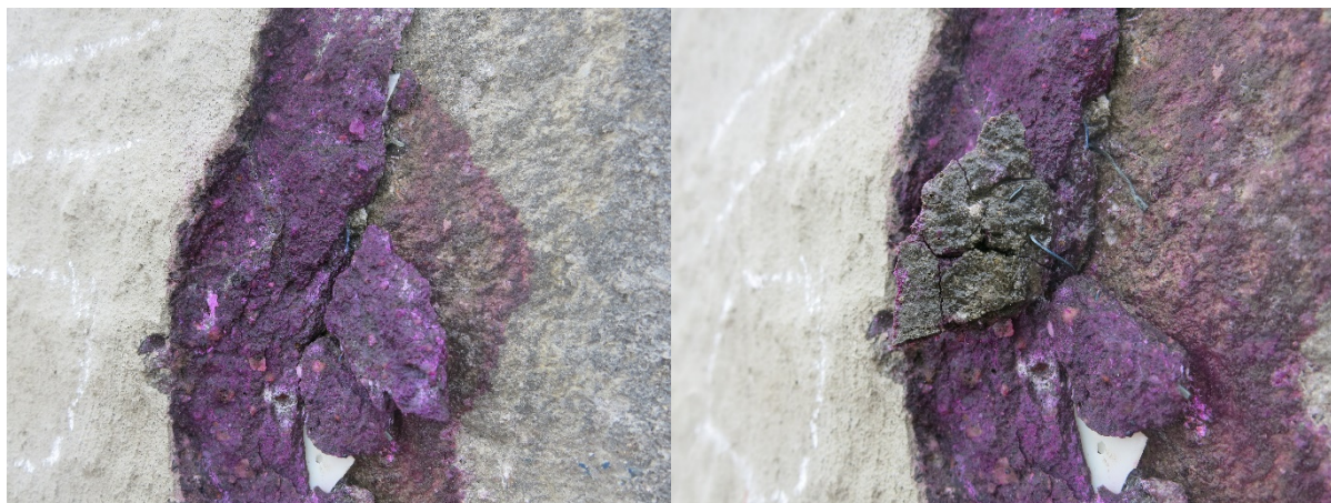
Figure 5-2 Delaminated area sprayed with phenolphthalein.
