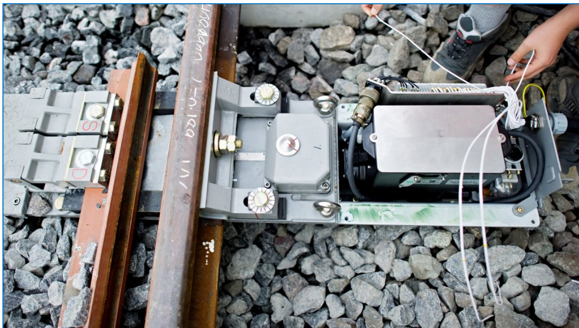
Figure 20: Switch monitoring. (Source: Banenor.no (2019))
