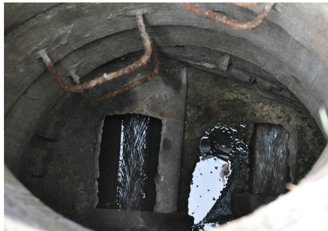
Figure 1.4 Combined manhole can be a source of unwanted water I/I in separate sewers.
