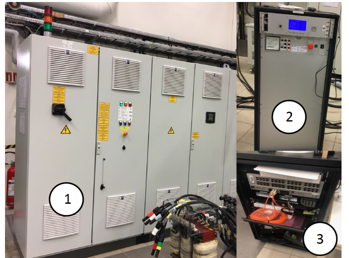
Fig. 9. Norwegian Smart grid Laboratory. (1): 200kVA Controlled Voltage Source, (2): 60 kVA 3 - \phi VSC, (3): OPAL-RT.
