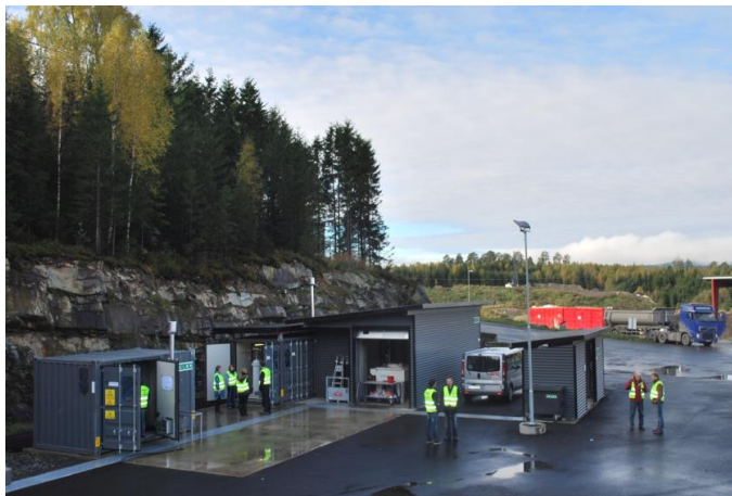
Figure D.7: Biogas upgrading plant at Glør IKS, Lillehammer, Norway
