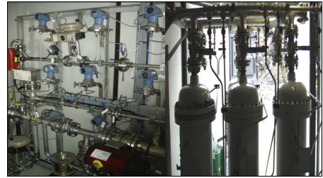
Fig. 4. Photographs showing the biogas upgrading membrane plant.
