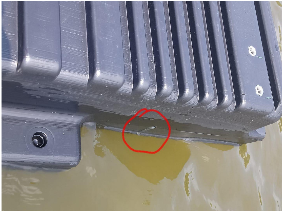
Figure 24. Unplugged up injection hole on floating module.
