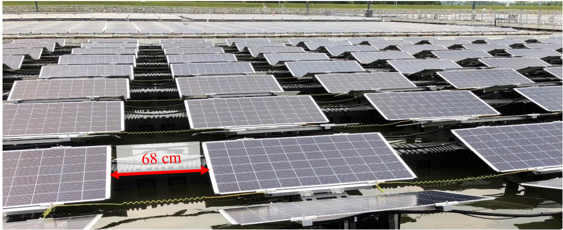
Figure 23. Gap between PV panels.
