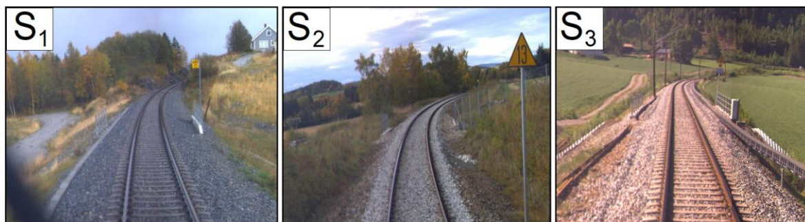
Figure 5.3 – ROGER 1000 photos at the site conditions at S 1 ) Sjånes, S 2 ) Holme and S 3 ) Viker culvert
