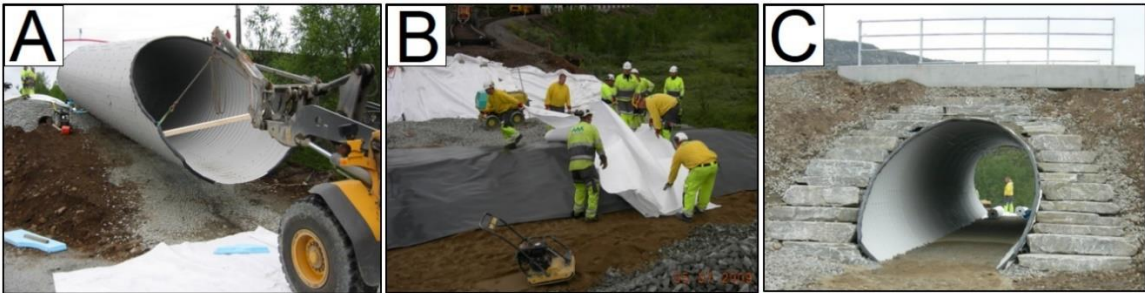
Figure 1.12 – Installation and construction of Solheim culvert in 2009 during a short traffic stop (Source: ViaCon Norway)
