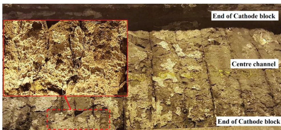
Figure 4.50. Cathode surface of pot 5 showing a relatively uniform wear. Highlighted spot illustrates the occurrence of pitting.
