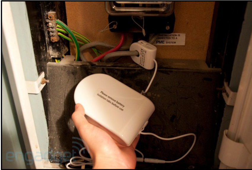
Figure 21: There is no need for a smart meter when using AlertMe [19]
