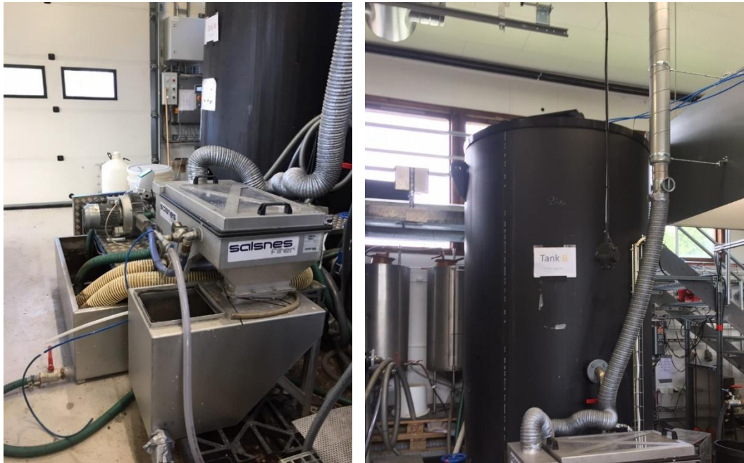
Figure 9: Salsnes filter and Wastewater tank
