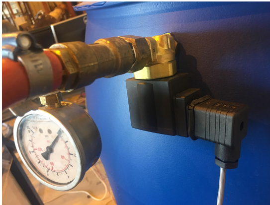
Figure 9.17: Solenoid Valve installed on the tank
