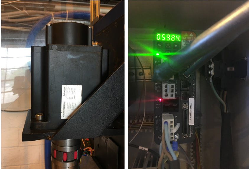
Figure 9.6: Servo motor and its drive installed on the rig
