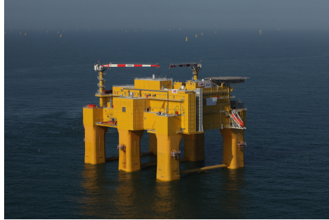
Figure 2.4: ABBs DolWin 2 offshore converter station [27].
