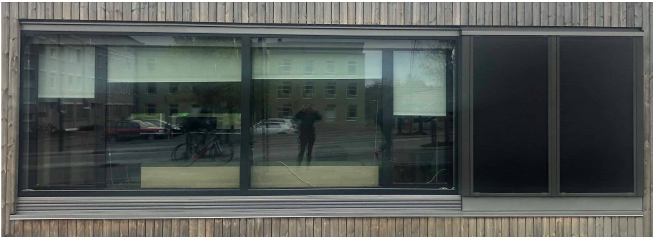
Figure 6.5: South facing windows with solar thermal collector, Living Lab
