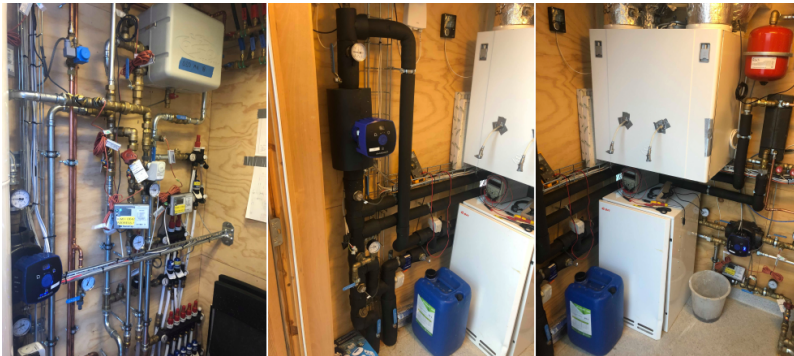
Figure 5.3: Inside the technical room in Living Lab
