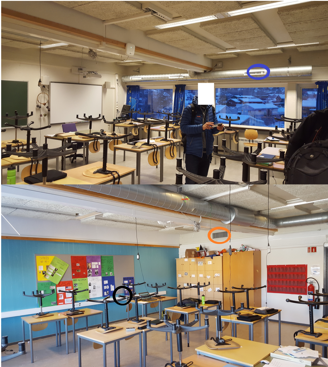
Figure 9: Pictures from Room 207. The supply air iButton is marked by a blue circle, the extract air iButton is indicated by an orange circle and the ELMA monitor by a black circle. The ELMA monitor had been removed before the bottom picture was taken.
