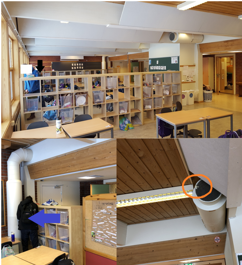
Figure 17: The ELMA monitors position is indicated by the a black arrow. It was placed in the second row of open shelves seen in the top picture. The displacement diffuser with the supply air iButton is seen in the back of the top picture and in the bottom left picture. The supply air iButton was hidden behind the diffuser indicated by the blue arrow. The orange circle marks the extract air iButton. (Credit bottom pictures: "Skoler på vent")
