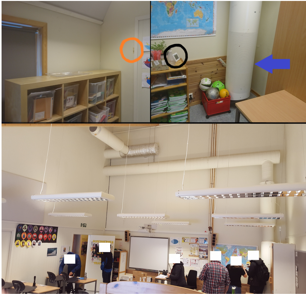
Figure 16: The top left picture shows the "extract" air iButton, marked with an orange circle, taped on wall in the back of the classroom. The top right picture shows the positioning of the ELMA monitor (black circle) and the displacement vent with the supply air iButton taped on the backside, indicated by a blue arrow. (Credit top pictures: "Skoler på vent")
