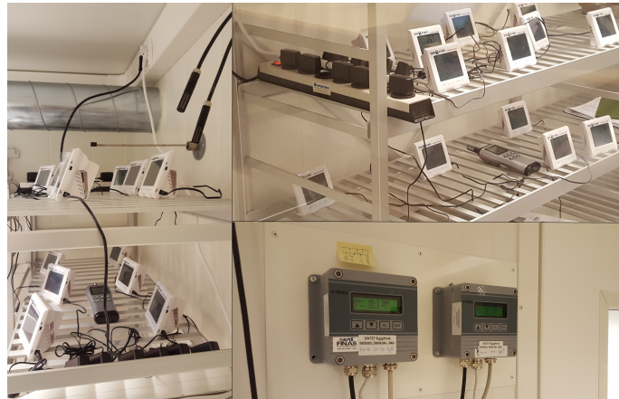
Figure 1: The picture to the left shows the setup for Room 2. The two black rods are the permanent room sensors. The top right picture shows the setup in Room 1. The bottom right picture illustrates the two permanent sensors in Room 1.
