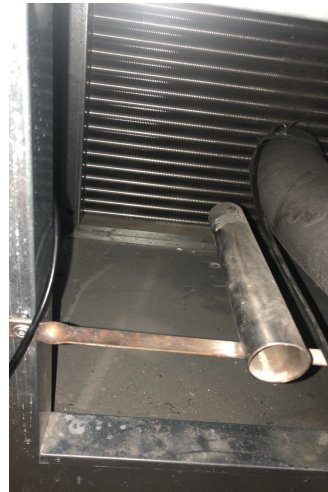
(b) The exhaust inlet room
