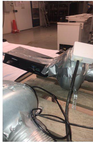
(b) Sensor connected to the supply fan
