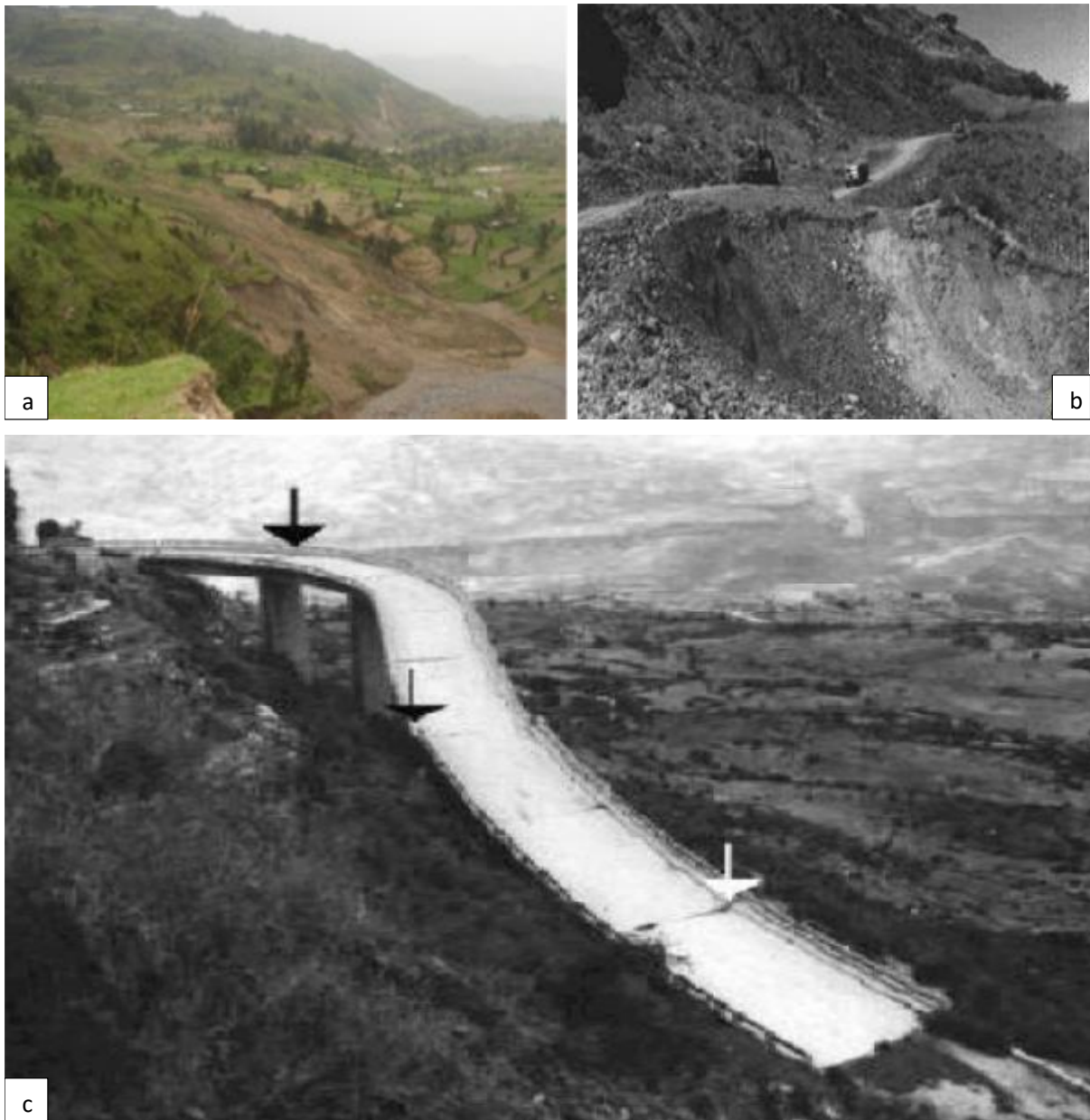
Figure 2-2 (a) Large-scale rockslide and associated debris/earth slides/flows on volcanic terrains, Tarmaber area, central highlands of Ethiopia. (Woldearegay, 2013); (b) a road section damaged in August 1993; (c) Damaged bridge due to landslide in the Blue Nile basin (Ayalew, 1999).
