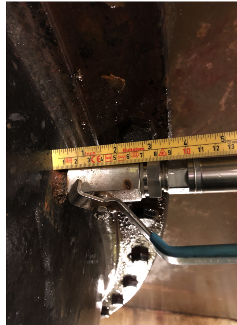
Figure 10.3: Picture of pressure transducer placed on the draft tube of turbine 1.
