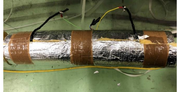
b) The Armaflex pipe insulation was covered with self-sealing fiberglass pre-slit pipe cover.
