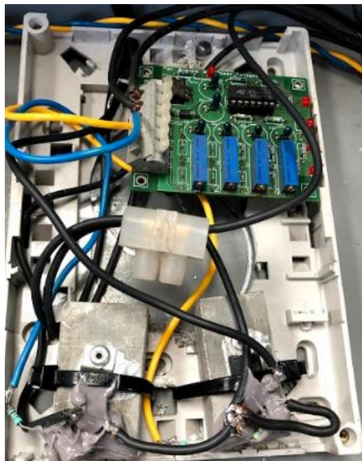
Figure 29: The actual controller box. The controller board at the upper part and the two switches with the connected resistors and aluminum below
