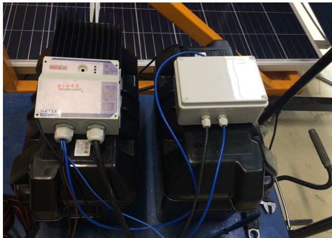
Figure 63: Battery setup with controller and fuse box
