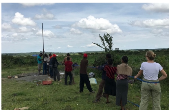
Figure 8.2: A lot of people had to help out when lifting up the rising main during reparation of an India Mark II Extra-Deep Well.
