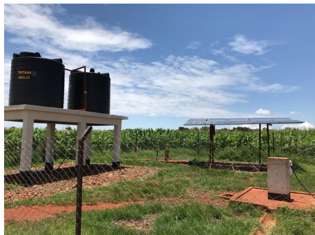
Figure 7.2: Solar powered pump with storage tanks.
