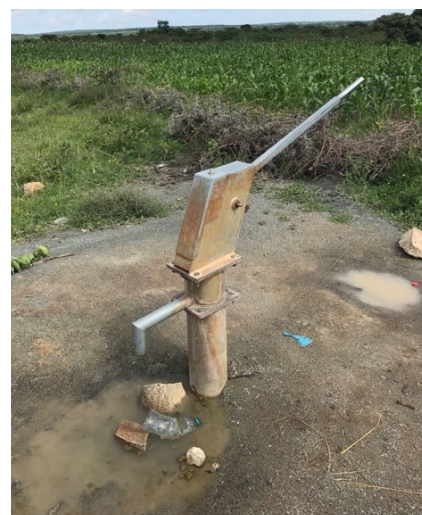
Figure 9.6: Hand pump in poor condition with both lack of fences and a concrete base.
