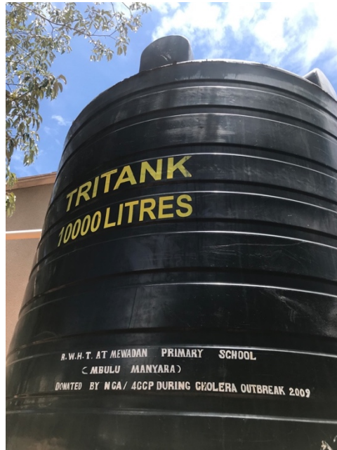
Figure 7.3: Rainwater harvesting tank at a school in Mbulu.
