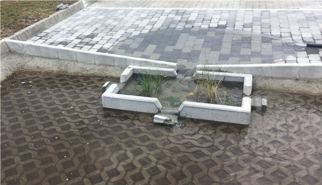
Figure A4: The main flow path noticed during the experiment, also illustrating the hose location, the inflow loss, the slope of curbs and the CGP overflow.
