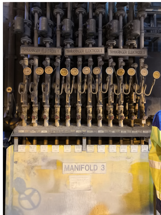
Figure 3.1: Manifold N3 at Elkem Bremanger (The photo is published with permission)
