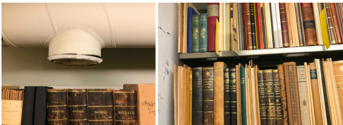
Figure 5.1: Visual inspection showing packed shelves and books located near the exhaust
