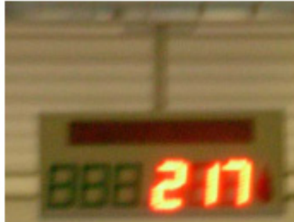
Figure 5- 5: Nurse Calling System with Electronic Boards in the Ceiling (Haug et al., 2004)
