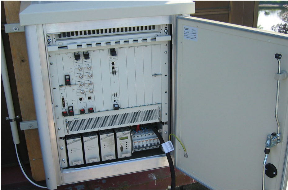
Figure 5.5: Base station installed in the cabinet at site BS1
