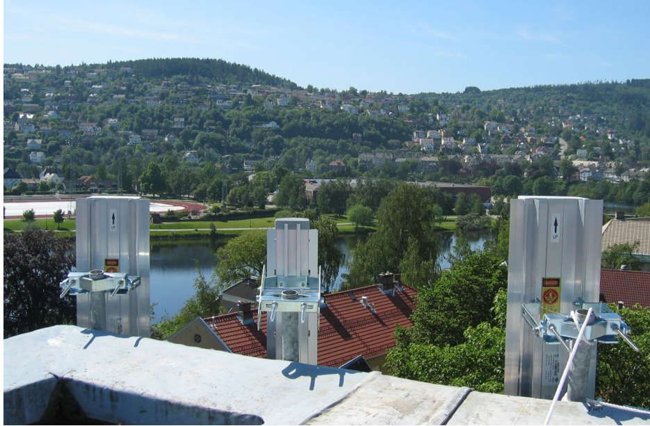
Figure 5.6: Antenna configuration at site BS1
