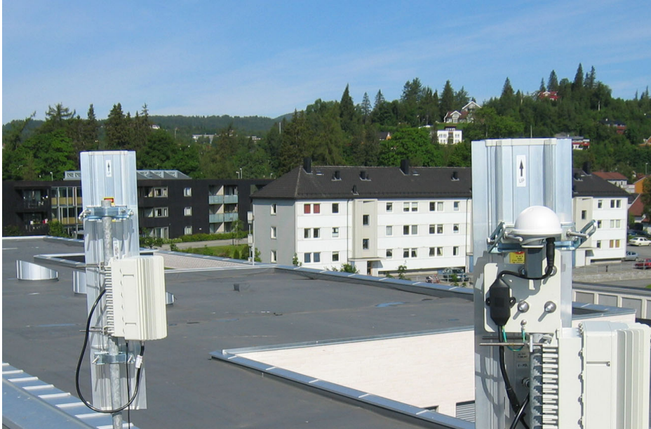
Figure 5.7: Antenna configuration at site BS2
