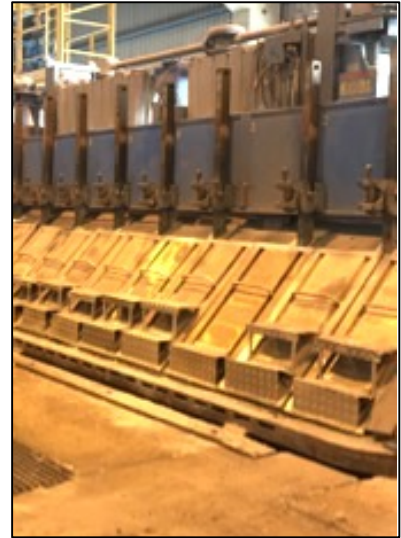
Figure 3.9: Damaged pot cover, missing the entire second step.
