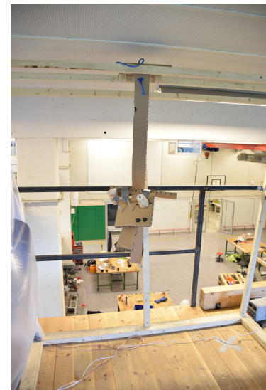
Figure 13: Second ceiling console.
