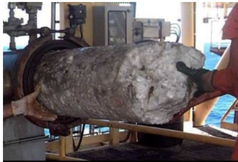
Figure 2.1: A large gas hydrate plug formed in a subsea hydrocarbon pipeline (Heriot-Watt University, 2017)
