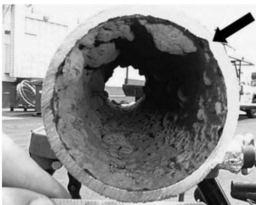
Figure 2.6: Pitting corrosion due to MIC in a carbon steel water pipe (Skovhus et al., 2017)
