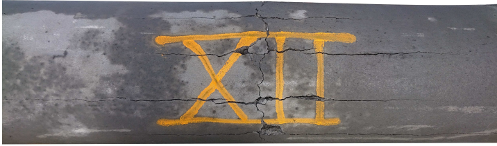
Figure 6.23: Characteristic crack pattern for reinforced concrete pipes subjected to blast loading (pipe XII).
