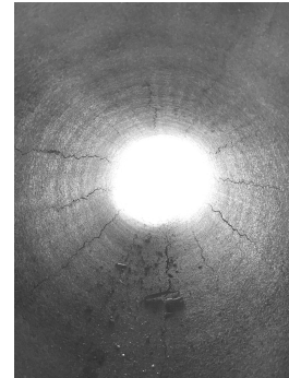
Figure 6.24: Through-thickness cracks in reinforced concrete pipe (pipe IV).
