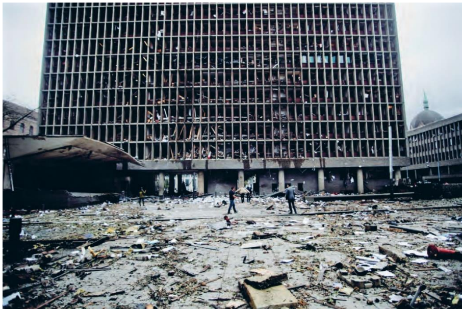
Figure 1.1: A high rise building in the Norwegian government quarter after the bombing on July 22, 2011, Photo by: Fartein Rudfford [1]
