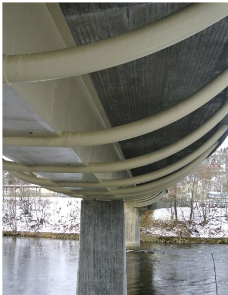
Figure 3.7 The underside of Cecilie Bridge with the steel beam and connection to the concrete slab.
