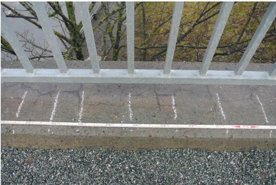
Figure 4.2 Another picture of the axis, the stirrups are marked. In this picture point 6.61 m is located, that is where later core B was drilled from. At 6.61 m the tiny 0.15 mm singular crack is hard to see, even on a close up picture. The cracks with a darker color is the map pattern type of cracks.
