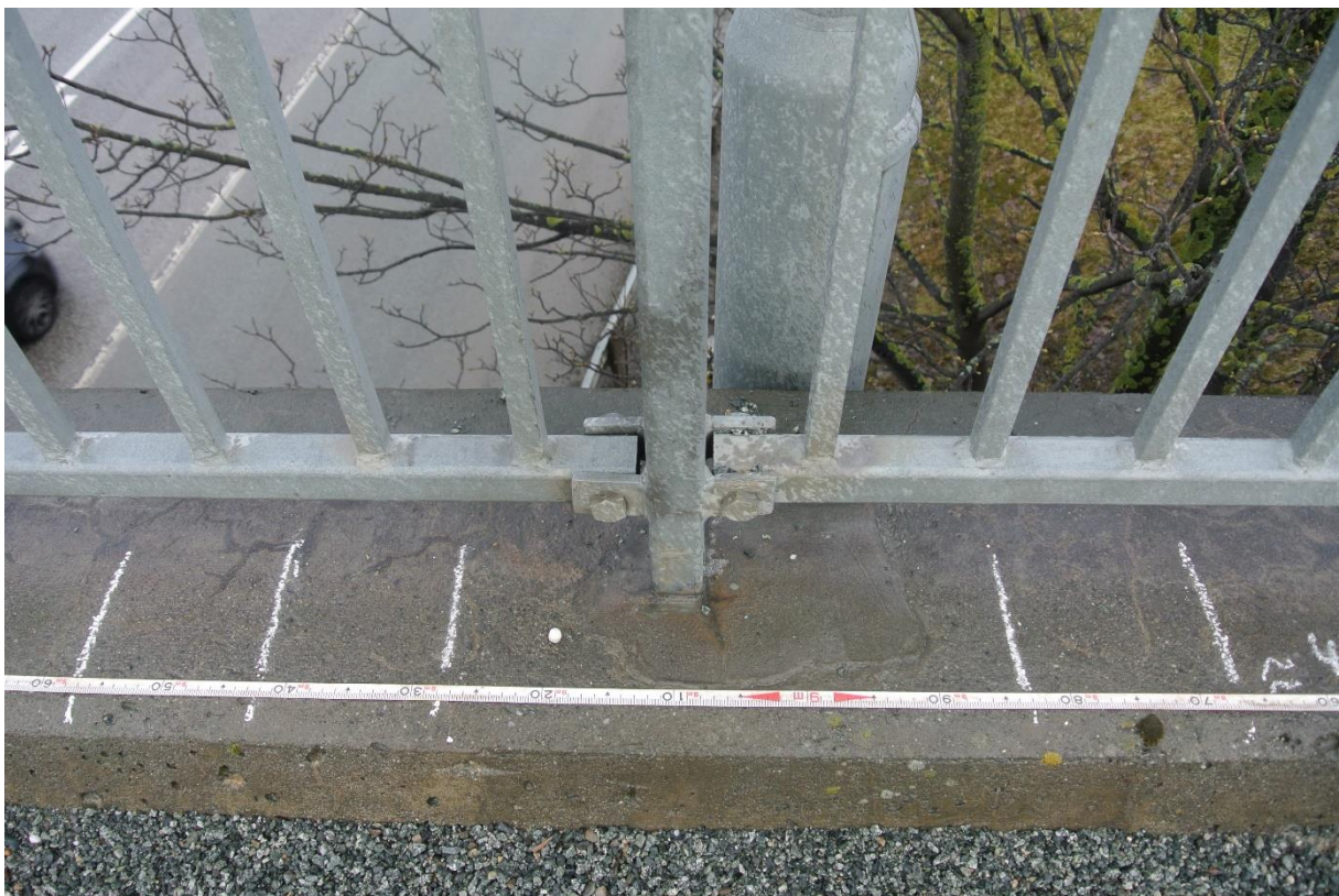
Figure 3.5 Fence post on Moholt bridge, extra concrete seem to be added around the post.
