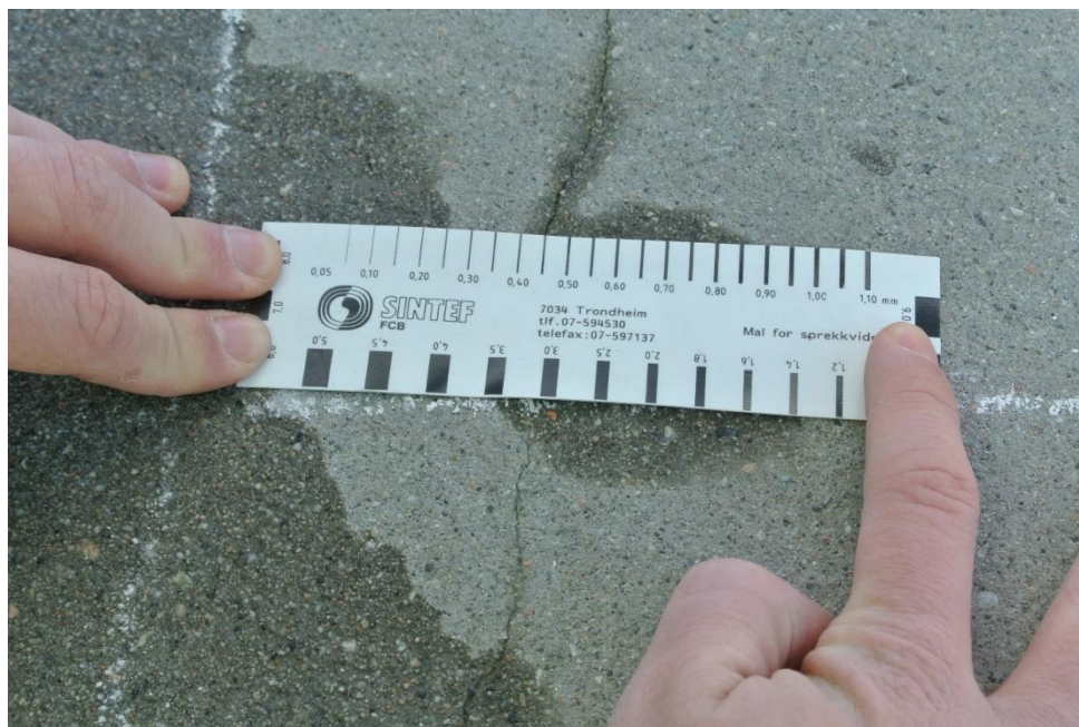
Figure 4.6 Measuring crack width where core A from Cecilie Bridge later was drilled.
