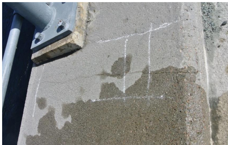
Figure 10.16: Investigated singular crack through the edge beam on Cecilie Bridge (Crack width 0.45 mm). Picture: Andreas Rygg
