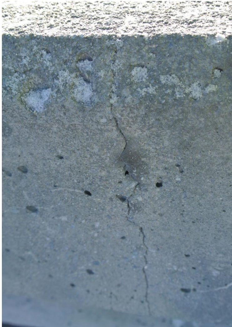
Figure 6.2 One of the singular cracks. This picture is from the outer side of the edge beam. This crack extends on the top surface to where core E was drilled.
