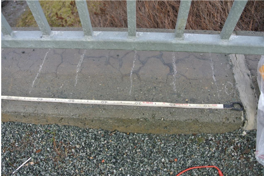
Figure 4.1 Point 0.0 m for the established axis along the norther edge beam of Moholt Bridge is to the right in this picture. It's a little bit hard to see in the picture, but the measuring tape follows the the 45-degree edge bevelled by a 20 mm lipping.
