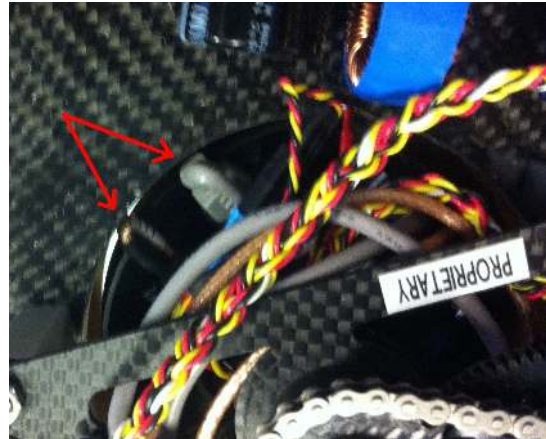
(b) The cables touching the mounting plate.
