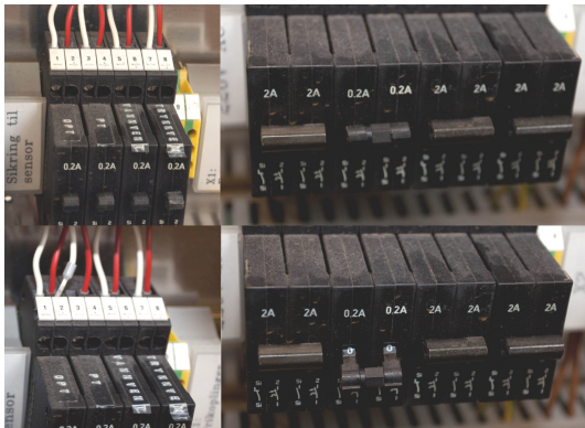
Fig. 5. Examples of error markers: normal cable (top left), loose cable (bottom left), normal fuse (top right) and tripped fuse (bottom right)
