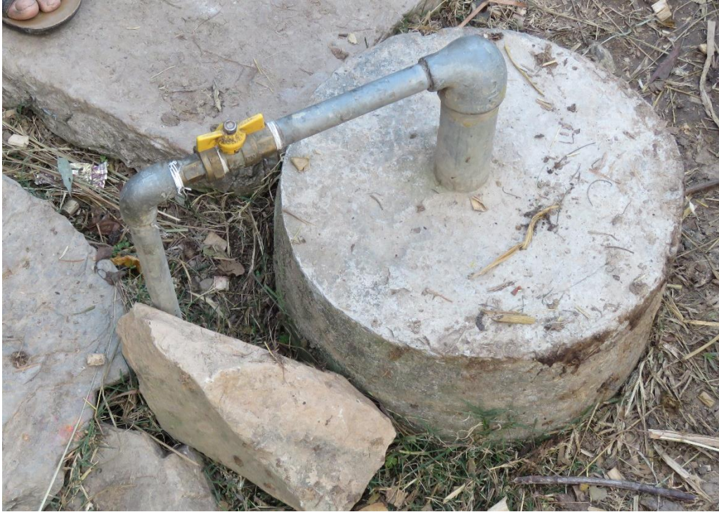
Gas valve which releases the gas into the home containers which is then used for cooking.
