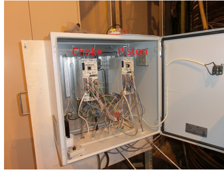
Figure 9: Inverters controlling the electrical motors
