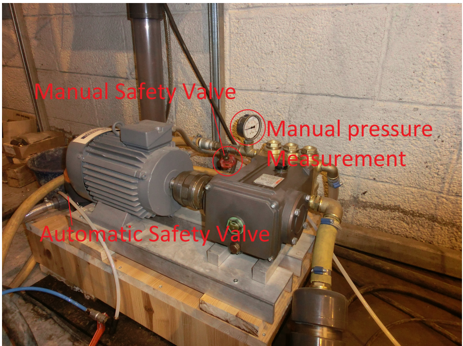
Figur C.10: Backpressure pump with the pressurizing valve.
