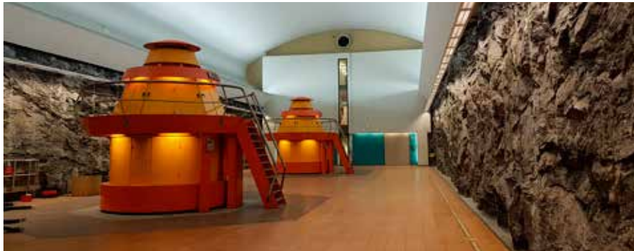
Duge power station with the two 100 MW reversible pump turbines
