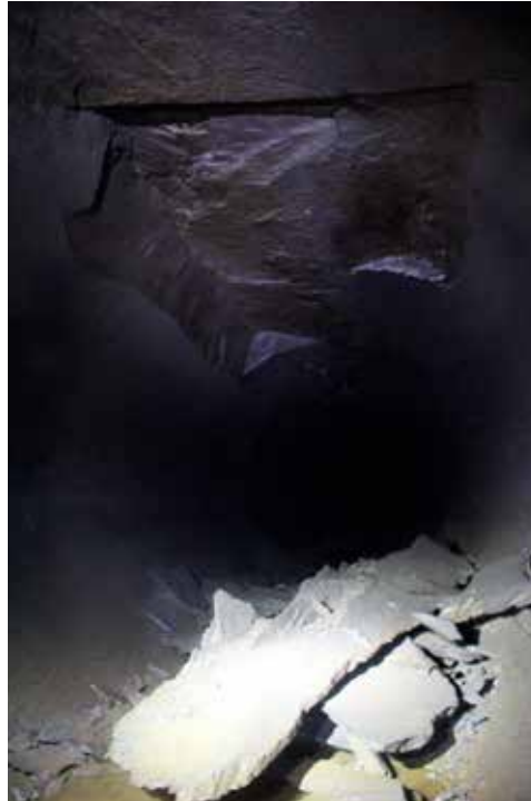
Rock fall in the roof of the headrace tunnel, caused by unfavorable joint systems and stress induced fracturing.
