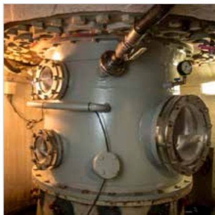
Plexiglass windows are installed on the draft tube of Svorka power plant (25 MW), operated by Statkraft
