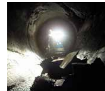
Block fall in the headrace tunnel in 2015, caused by joints and stress induced micro-cracking
