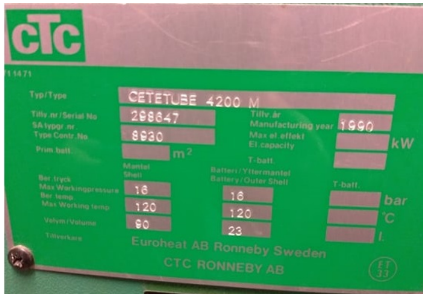
Figure 9: Nameplate of the heat exchangers at the NHL building.
