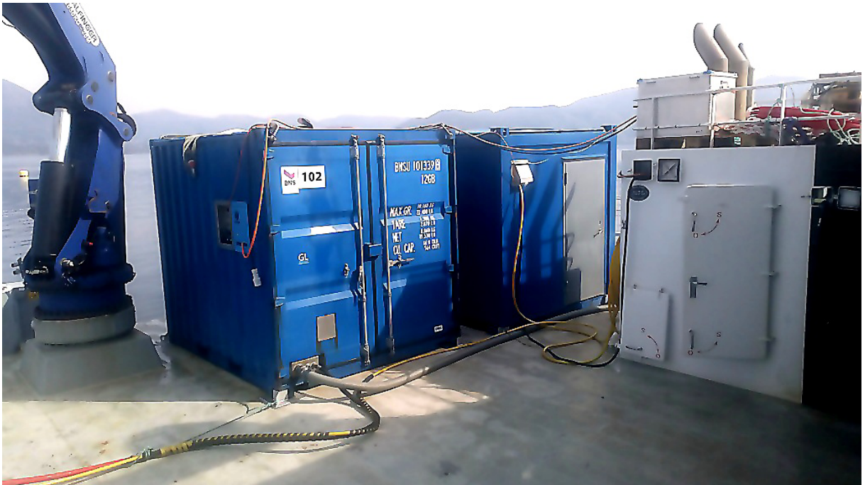
Figure 30: The containers that house the net cleaner system and the control room
