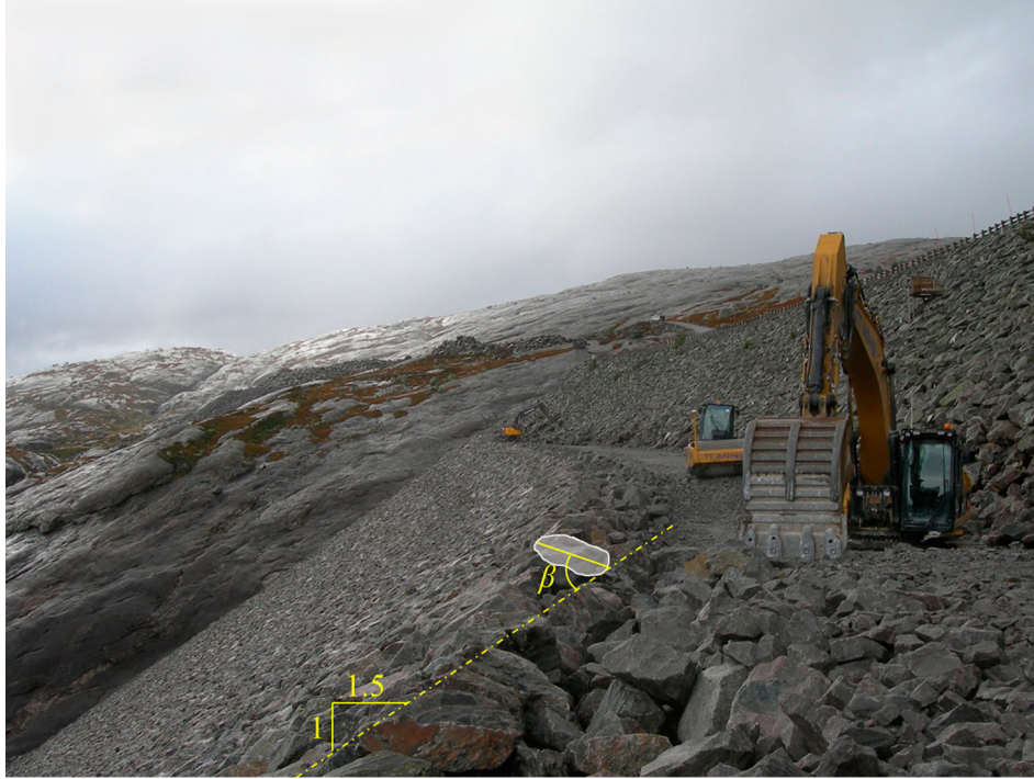
Figure 1. Rehabilitation work on the 129 m high dam Svartevatn in Norway. The riprap stones on the downstream slope are placed one by one in an interlocking pattern with their longest axes inclined towards the dam. The inclination angle \beta is the angle between the longest axis of a stone and the slope as indicated in the picture. (Photo NTNU).
