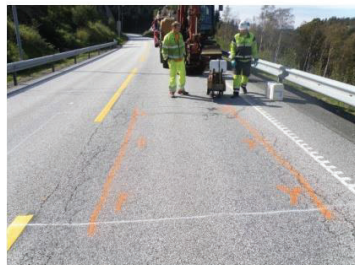
site II (damaged)
