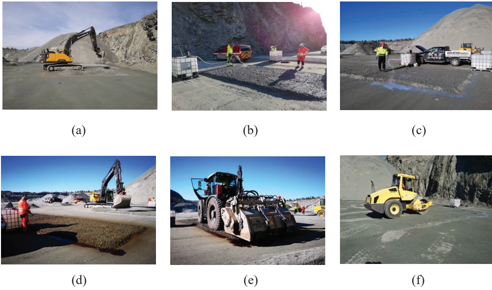
Figure 47 Construction of the first 15-cm part of the base layer: laying of the material (a), spreading water (b), spreading polymer-based additive (c), spreading lignin-based additive (d), mixing (e) and compacting (f)
