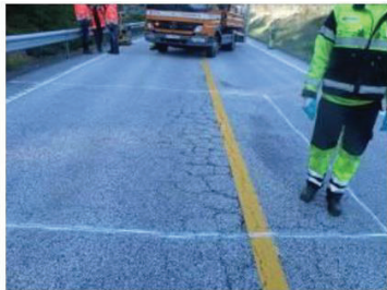
site I (damaged)
