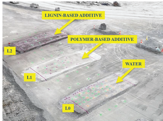
Figure 48 Construction completion of the road base sections: with water (L0), with polymer-based additive (L1) and with lignin-based additive (L2)
