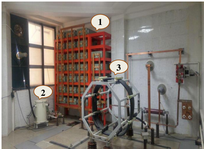
Fig. 2. Experimental Setup including: (1) Capacitor Bank, (2) Charging Circuit, (3) Reactor
