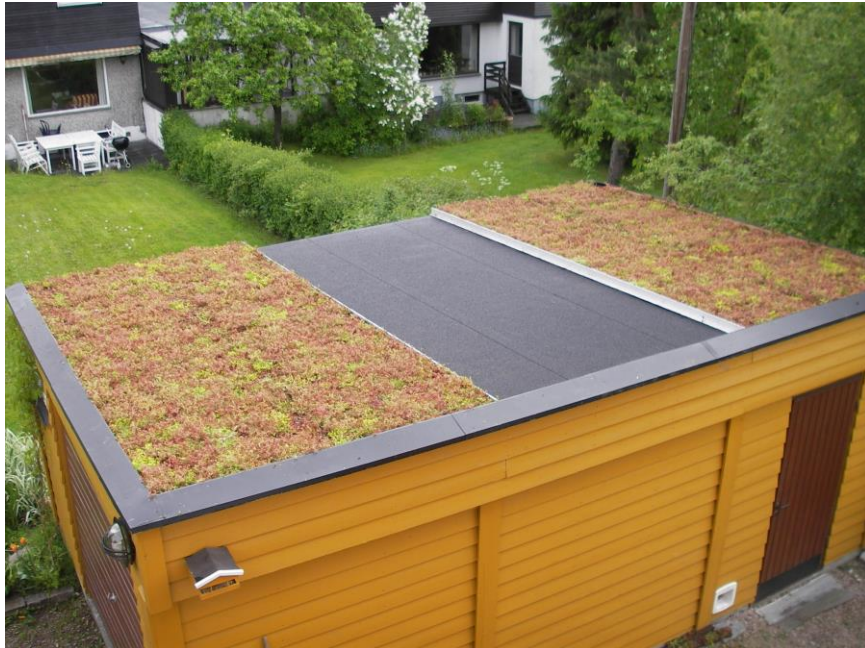
Figure A.1 GR1 (right), reference roof (RR) and GR2 (left). Photo taken when the roof was newly established in August 2009. Photo: Bent Brakserud
