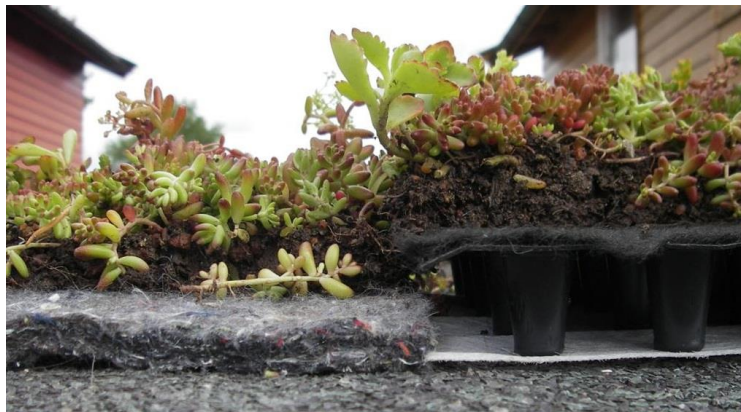
Figure A.2 Build-up of GR2 (left) and GR1 (right). Note that a VT-felt similar to GR1s was added to GR1 in August 2011. Photo: Bent Braskerud
