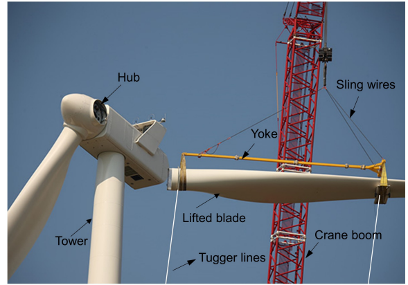
Figure 2: Image of a wind turbine blade being prepared to mate with hub of a turbine (source: [13])
